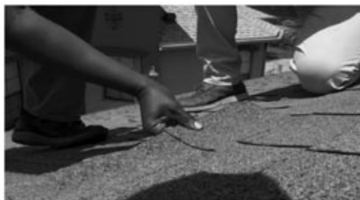
FREE Inspection and Estimate
