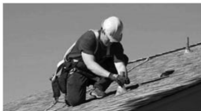
Make Necessary Repairs
